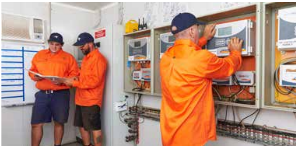
Irrigation Pump Station – Kingston Rest, WA
